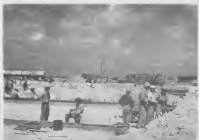
WORK is progressing at the plant site. Foundations are already dug and poured, and with the arrival of equipment, things are moving rapidly towards the completion date some time in 1958.
